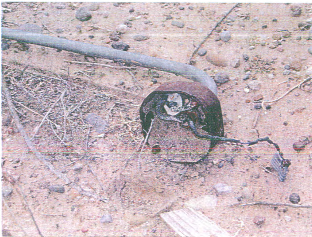
Figure 48. LA xx9, electrical wiring.
